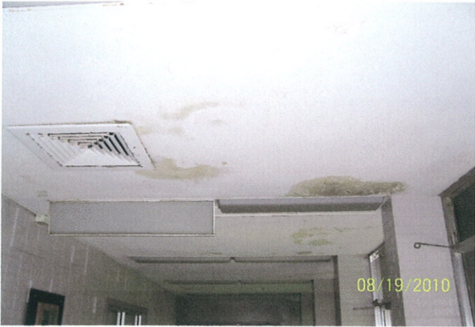
PICTURE#1- WATER DAMAGED PLASTER CEILING IN FRONT LOBBY/ENTRANCE
