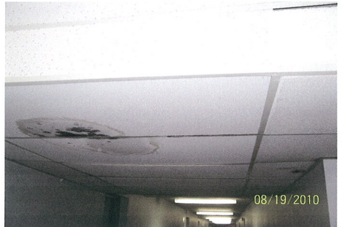
PICTURE#9-WATER DAMAGED CEILING TILE AND FUNGAL GROWTH IN BASEMENT CORRIDOR
