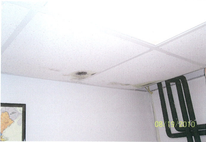
PICTURE#12- WATER DAMAGED CEILING TILES AND FUNGAL GROWTH IN PHOTO LAB
