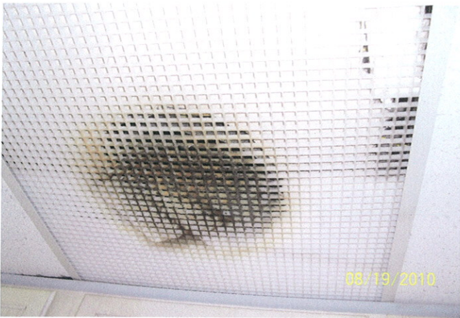
PICTURE#14-SUPPLY VENT IN BREAK ROOM IN BASEMENT
