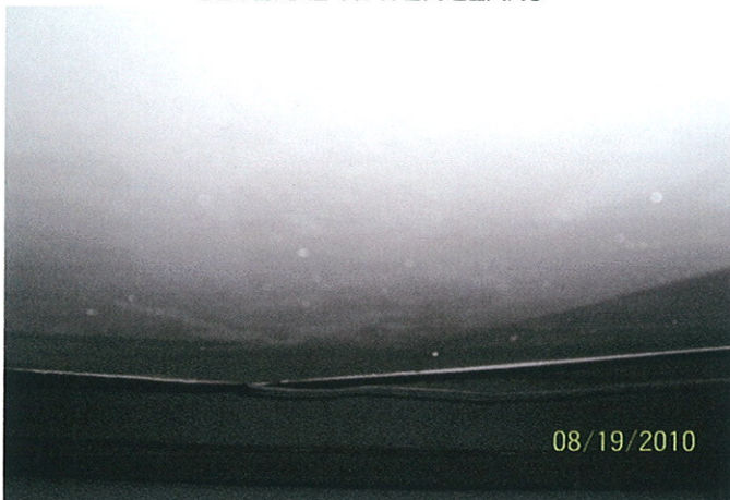
PICTURE#10-METAL DUCTWORK ABOVE CEILING IN PICTURE #9
