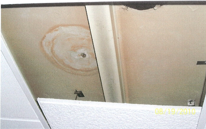
PICTURE#3-WATER DAMAGE-FIRST FLOOR CEILING-FRONT CORRIDOR
