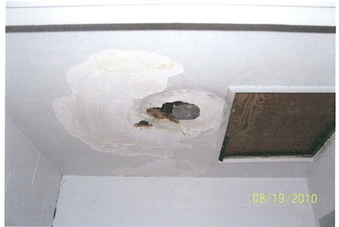
PICTURE#4-WATER DAMAGE-FIRST FLOOR MEN'S RESTROOM CEILING
