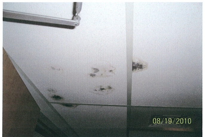
PICTURE#11-WATER DAMAGED CEILING TILES & FUNGAL GROWTH IN CSSU OFFICE
