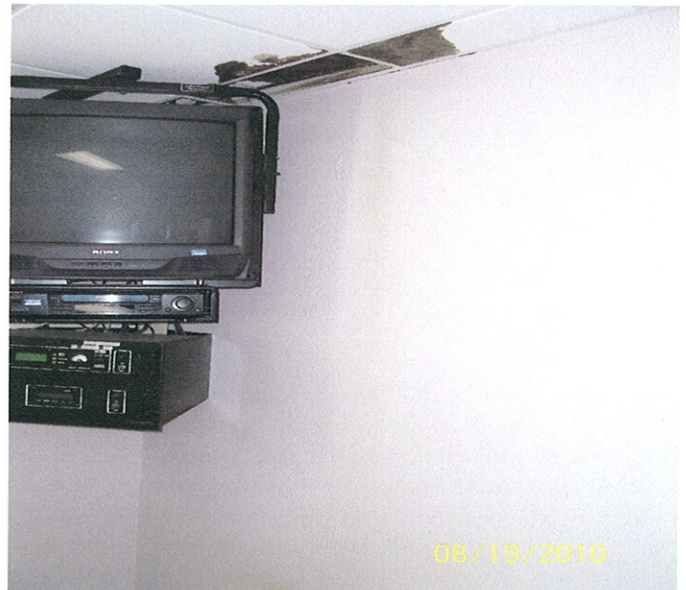
PICTURE#6-WATER DAMAGED CEILING TILES AND WALL IN ASSISTANT CHIEF OF POLICE'S OFFICE
