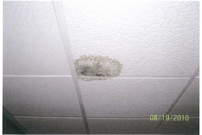
PICTURE#2-WATER DAMAGE & FUNGAL GROWTH- FIRST FLOOR CEILING-FRONT CORRIDOR
