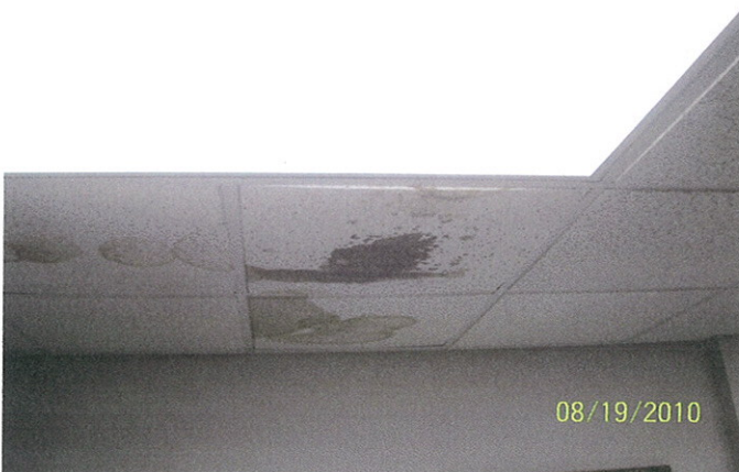
PICTURE#5-WATER DAMAGED CEILING TILES IN CHIEF OF POLICE-SECRETARY'S OFFICE
