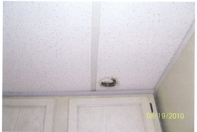
PICTURE#15-WATER DAMAGED CEILING TILE & FUNGAL GROWTH IN BREAK ROOM IN BASEMENT
