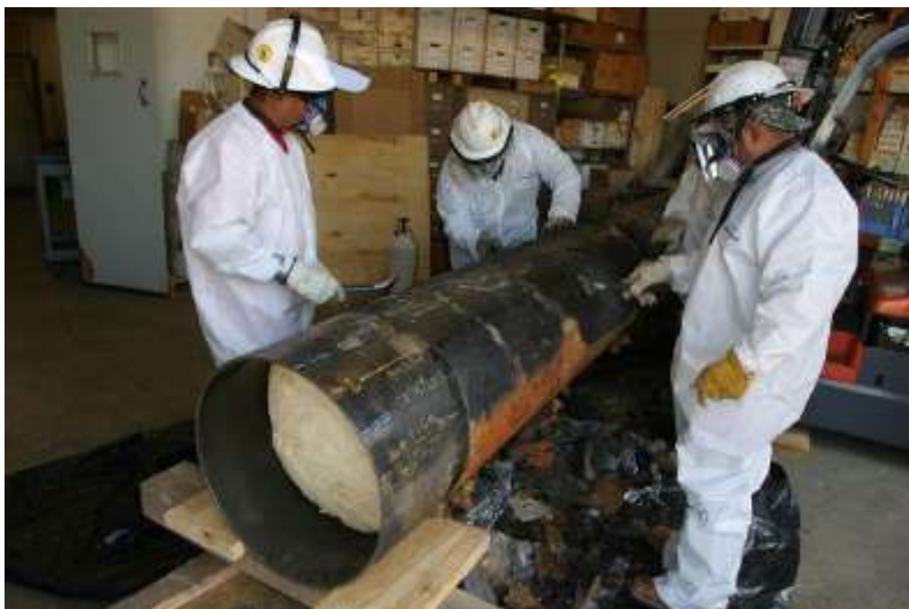
The photographs display the hand removal process of the coating which remained on the pipe after initial removal with hammer.
