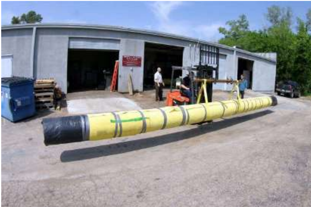
The photographs display two (2) pipe sections during the unloading process. There was no evidence of any transportation related damage to the pipe sections.
