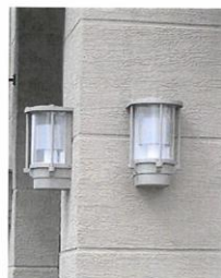
Building Sconce Lighting
