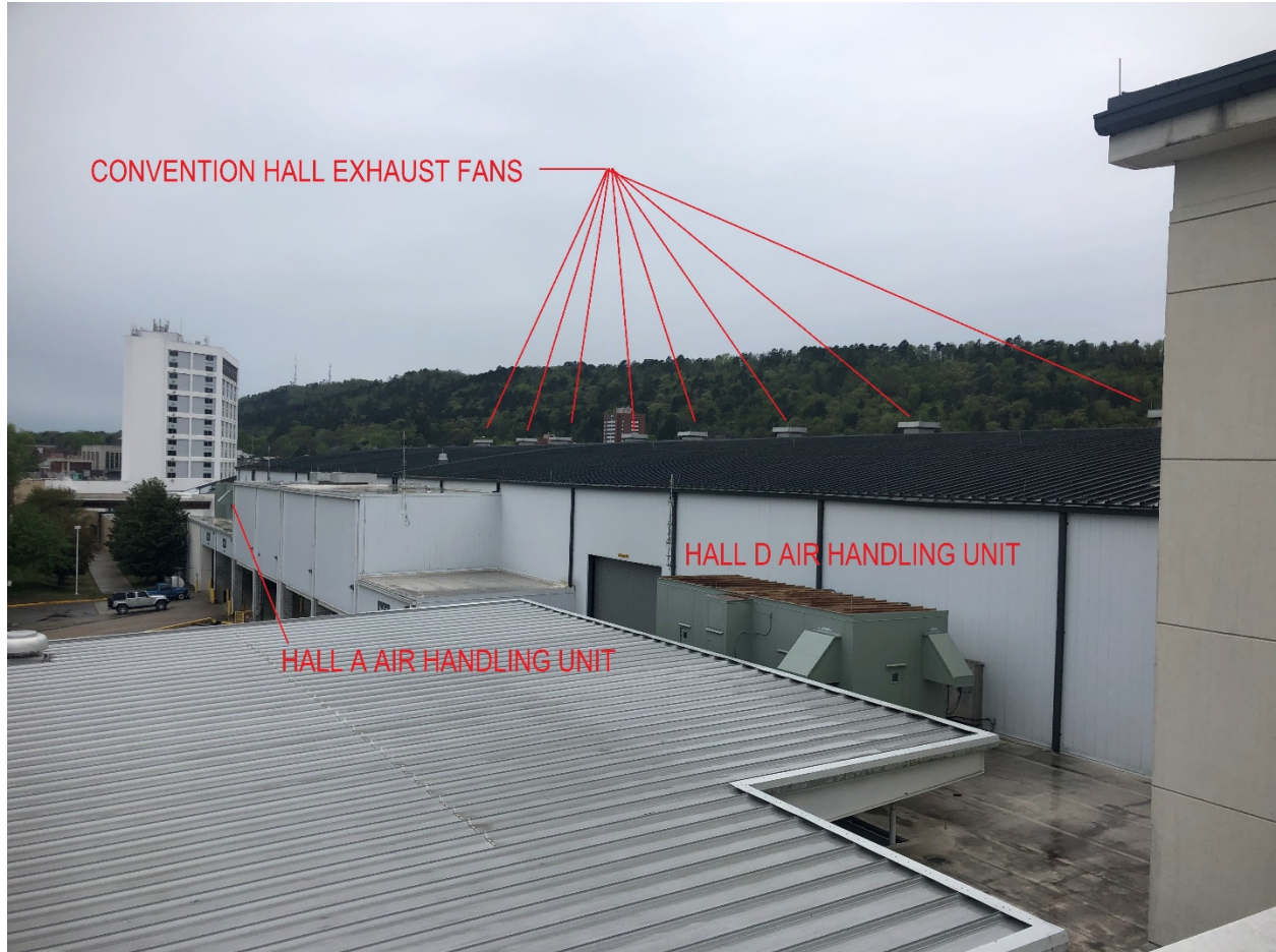
CONVENTION HALL HVAC UNITS
