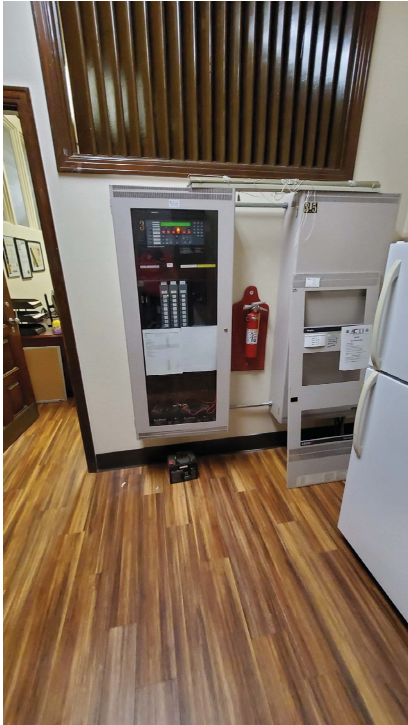
FIRE ALARM PANEL
