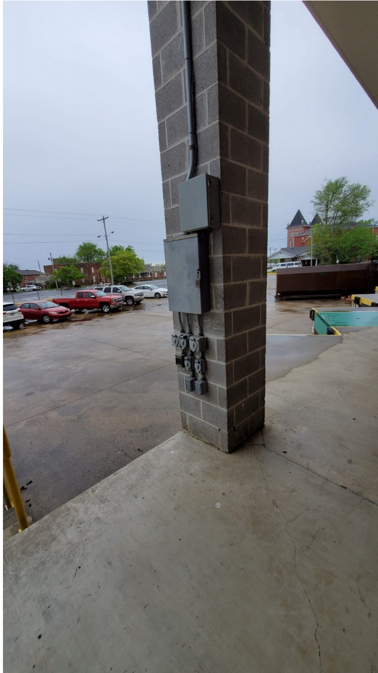
EXT. POWER AT LOADING DOCK
