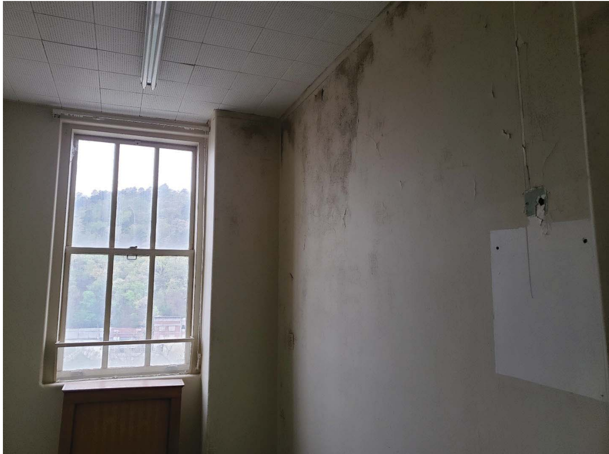
MOLD IN ROOM
