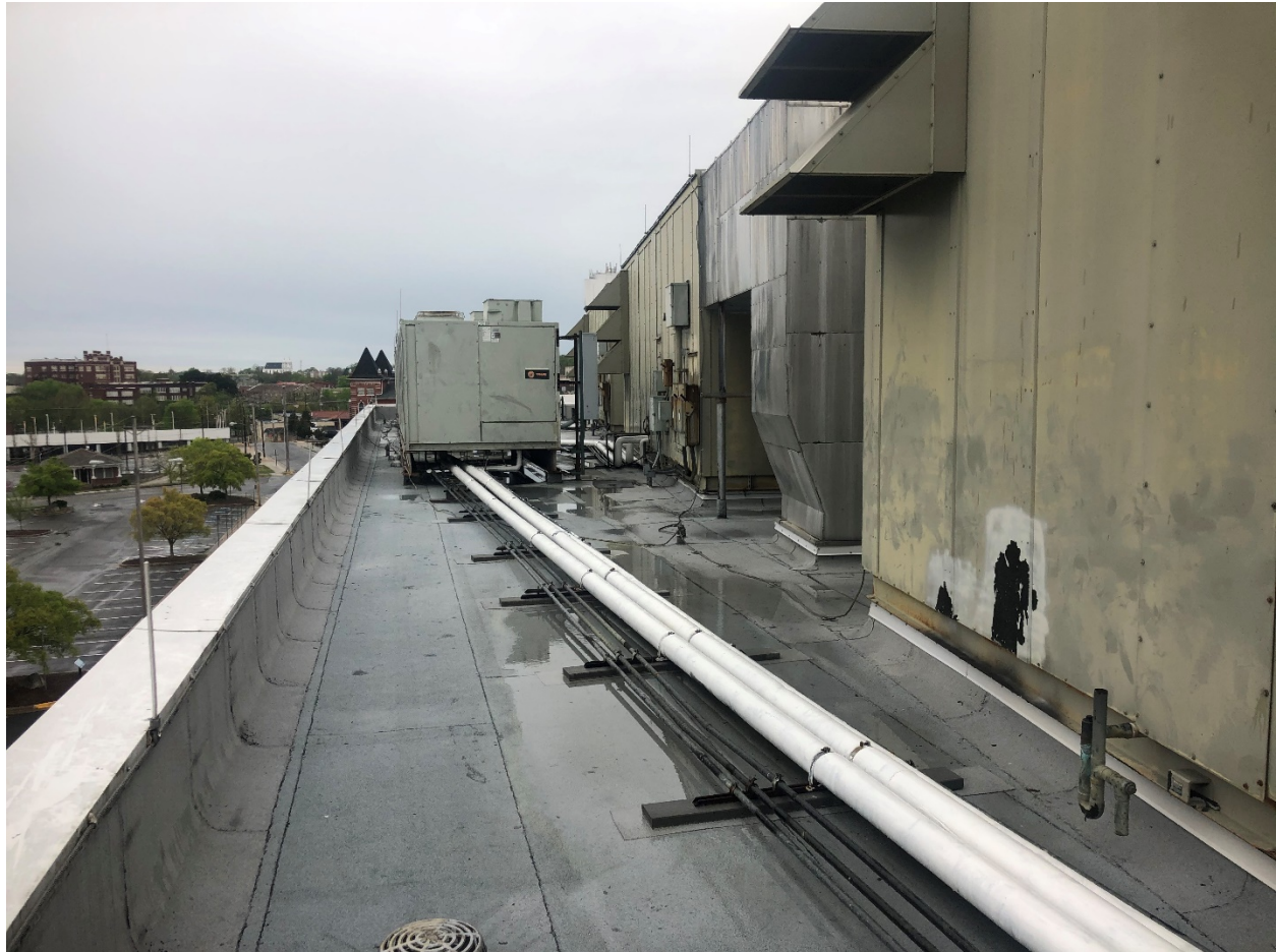
ENERGY RECOVERY UNITS AND OUTDOOR UNITS SERVING THE ARENA
