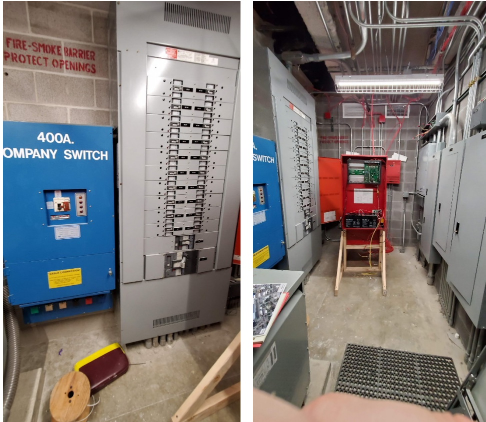
ARENA ELEC RM. COMPANY POWER AND SWITCHBOARD
