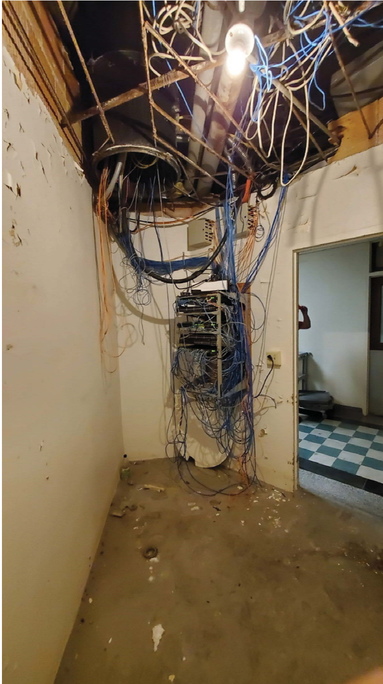
LAUNDRY CHUTE AND LAN RACK
