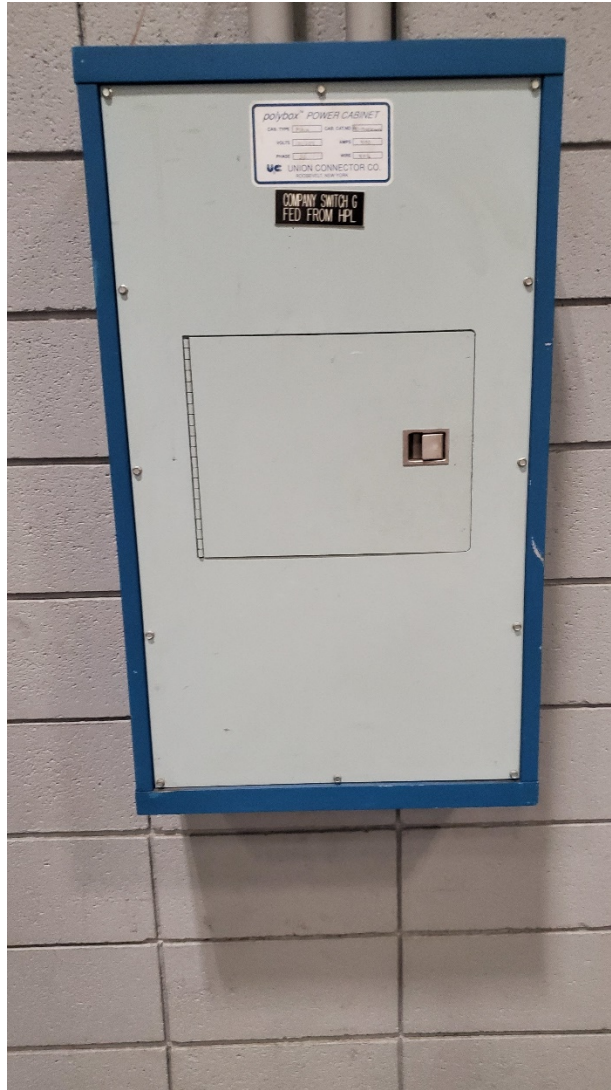
Figure 3: Company Power on Exterior Wall
