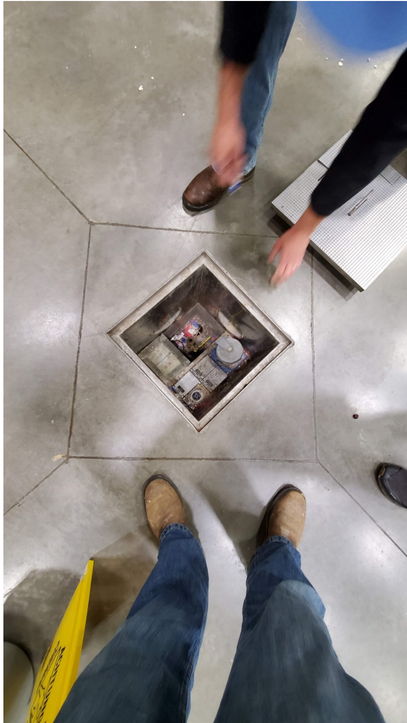
NORMAL POWER IN FLOOR AT ARENA
