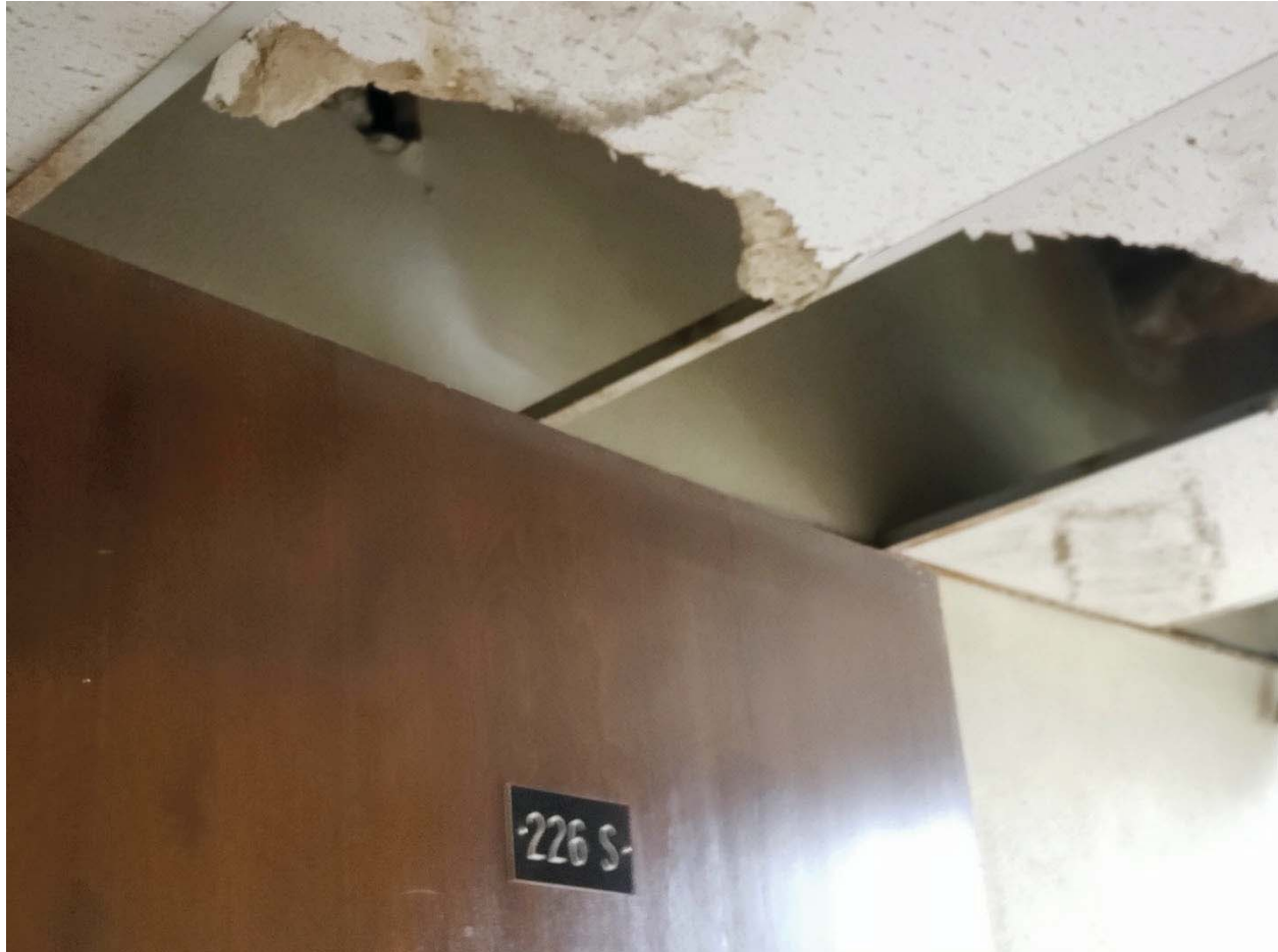
CEILING TILE WATER DAMAGE
