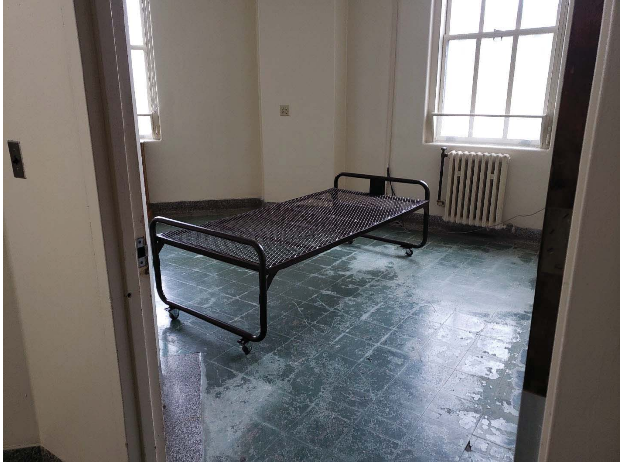
9x9 FLOOR TILE (LIKELY ASBESTOS)
