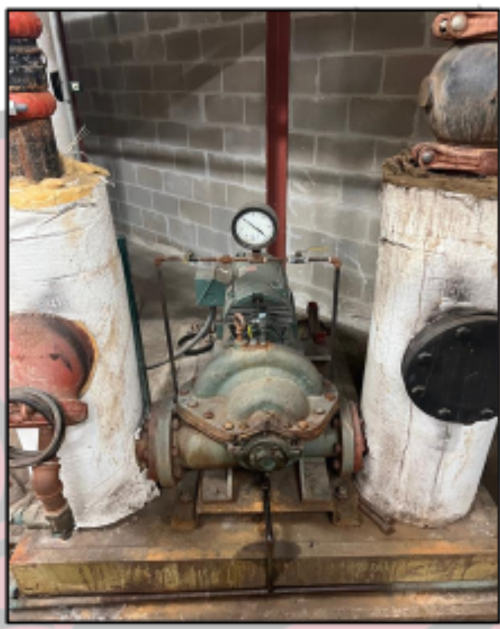
Badly aging Hot Water Pump
