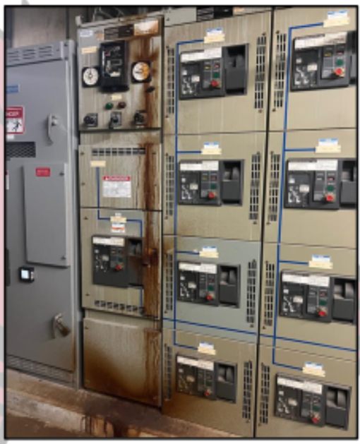
Electrical Entry Equipment with visible rusting
