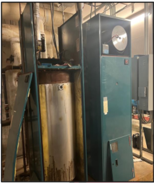
Inactive Boiler being cannibalized to keep the other 4 Boiler units operational
