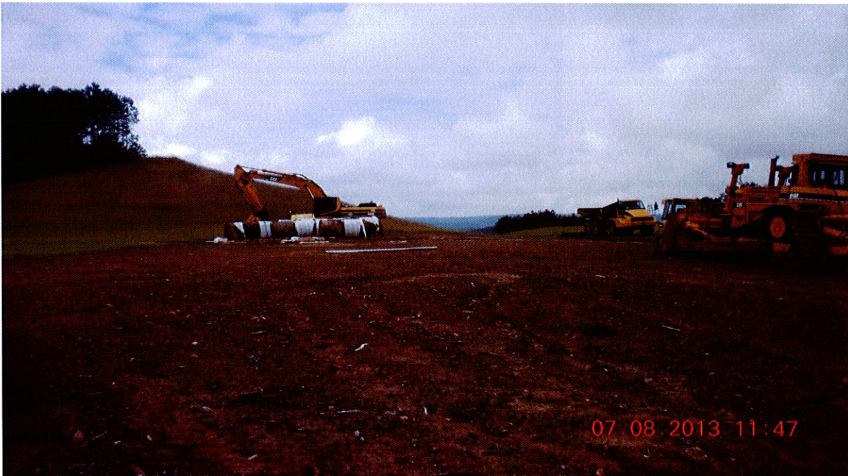
Photograph 8: Photograph showing the remaining equipment staging area. This area should also be stabilized upon project completion.
