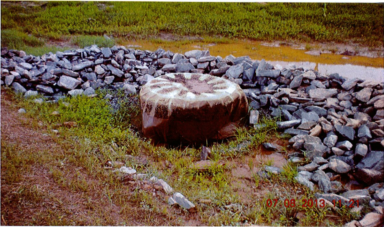
Photograph 7: Inlet protection device in need of maintenance.
