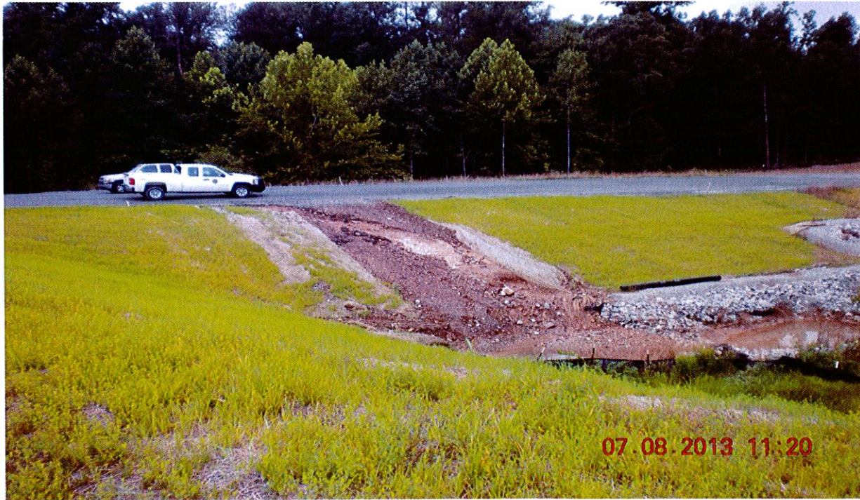
Photograph 6: Slope failure located near the end of the western roadside ditch in photograph 5. This area need to be re-graded and stabilized accordingly.
