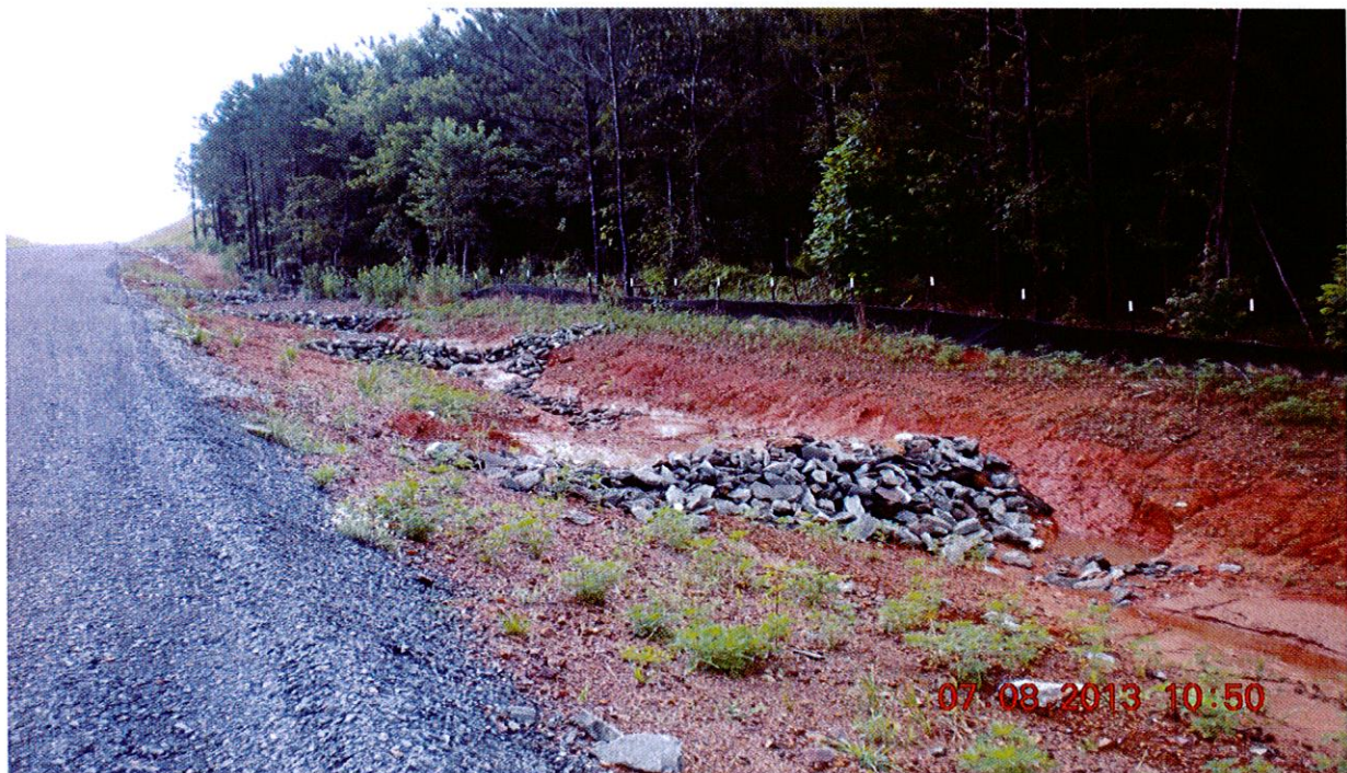
Photograph 4: Photograph showing check dams in need of maintenance/replacement. This photo also shows the eastern roadside ditch that must be addressed concerning post construction erosion issues.
