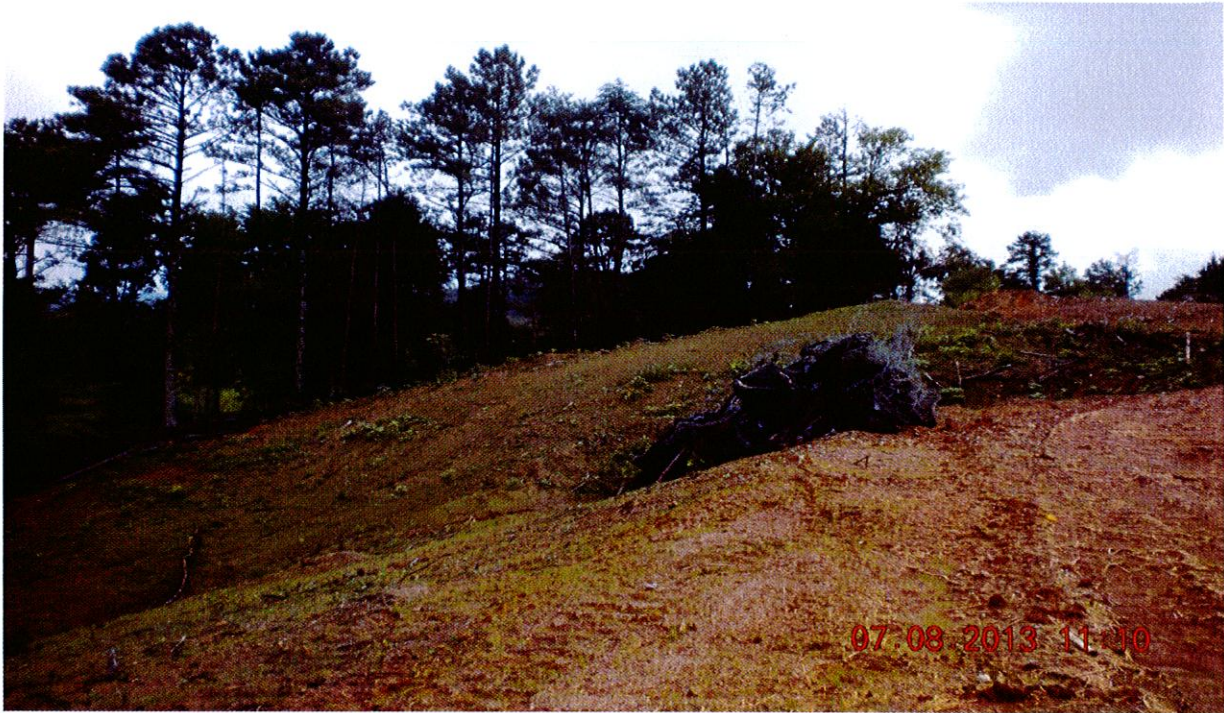
Photograph 1: Photograph showing steep slopes that have been hydro-seeded on one of the private inholdings of the project.
