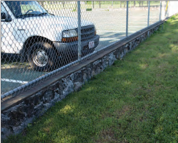
C. Detail of Southeast Wall of Tennis Court Foundation Showing Historic Rock Construction.
