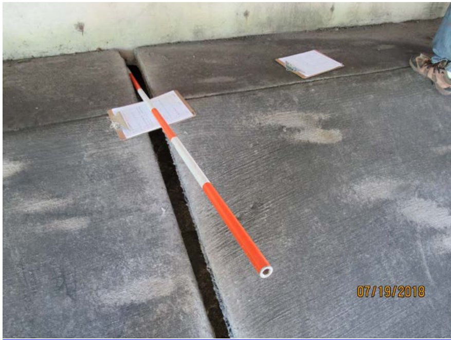
UNDERCUTTING - 8' ROD TO RESISTANCE - ABUTMENT 2
