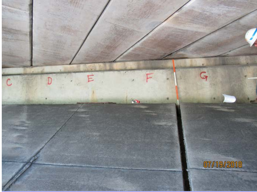
UNDERCUTTING - 4' ROD - TO RESISTANCE – ABUTMENT 2
